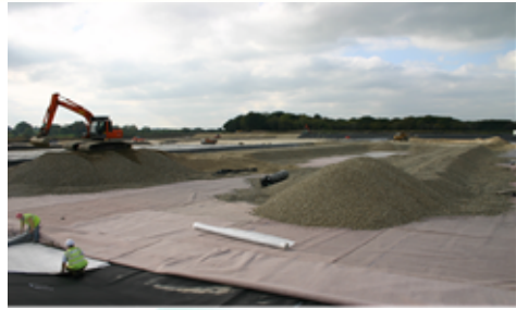
Connaught Regional Landfill – Drainage
