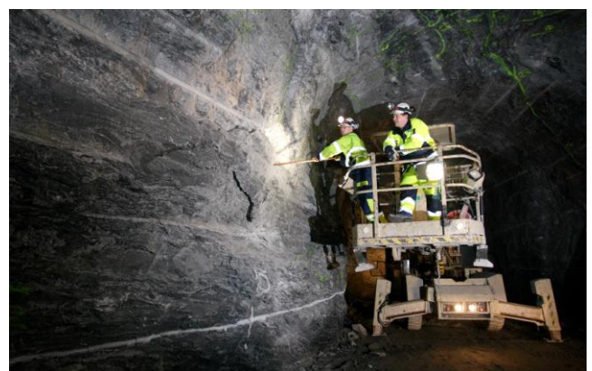
Construction of Posiva underground radioactive waste storage facility at Onkalo, Finland (courtesy of www.posiva.fi )
