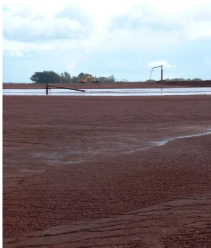
Mud discharge spigots and fresh flow at Aughinish Alumina
