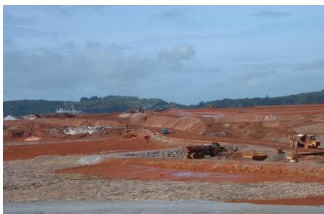
Looking west over the mud stack from the Aughinish plant site (straw on mud in foreground reduces dusting; dumpers carry salt cake to disposal area)
